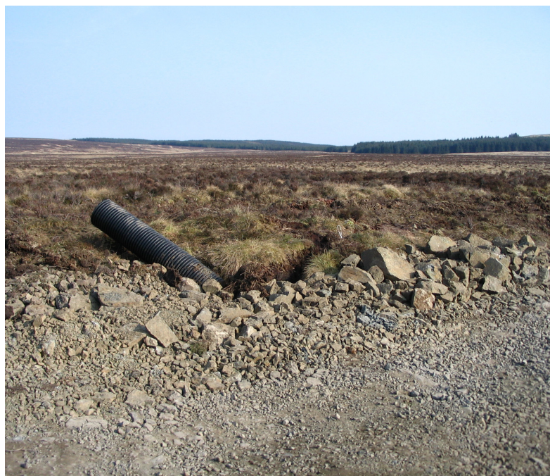
Figure 9. A floating road that has sunk and snapped the drainage pipe which was constructed to provide cross track water flow to mitigate for the hydrological impact of the track. Credit: Ian Thomas, SEPA.
