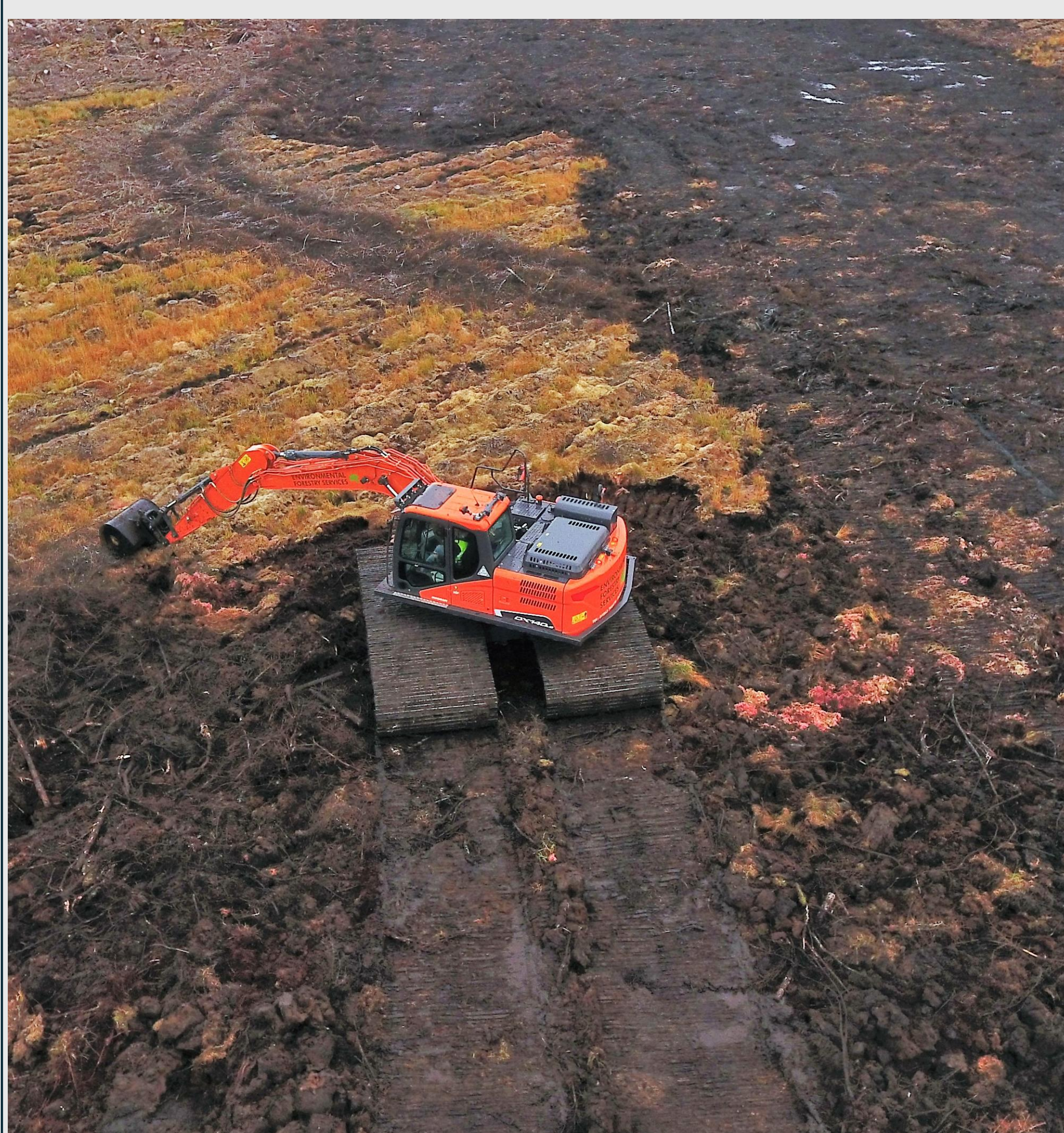
Figure 3. Contractors on 5-year contracts can invest in specialist machinery like this wide-tracked excavator being used for ground smoothing on a forest-to-bog restoration site. Operators gain expertise through working on many different sites and in turn they help refine techniques.
